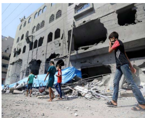
Gaza war damage photo by Mohamad Zaanoun, International Health Partners
